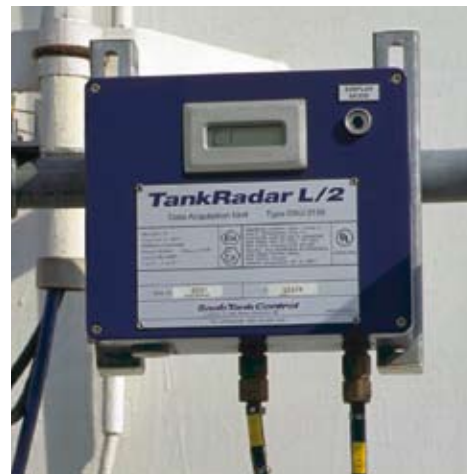
DAU with Local Readout display mounted at the foot of the tank.
